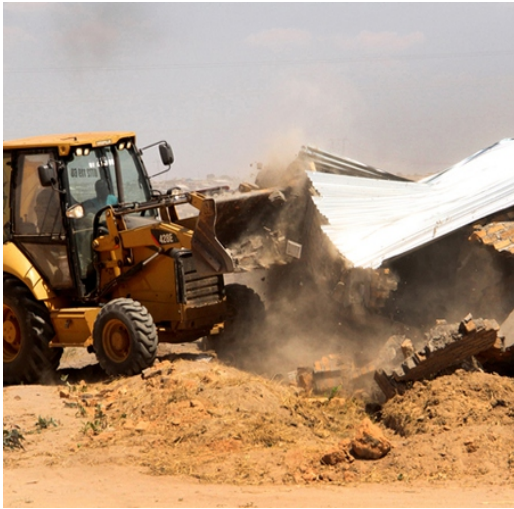
A bulldozer demolishes one of the illegal structures constructed on private property at Caledonia farm in Harare - Picture credit- Kudakwashe Hunda Source - Sunday Mail 2021
